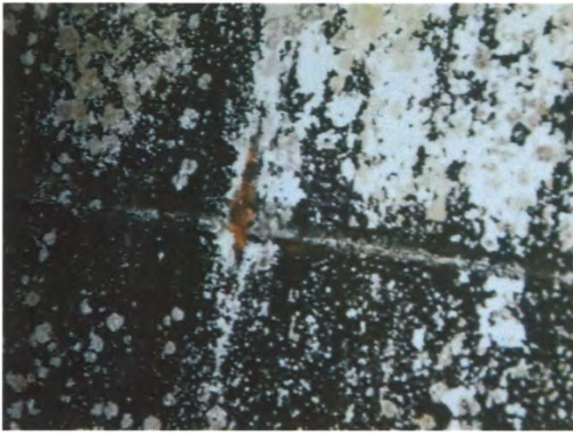
67 Interior Wall Having Coating Loss, Exposed Steel And Corrosion
