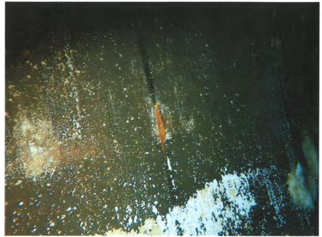
68 Interior Wall Having Coating Loss, Exposed Steel And Corrosion
