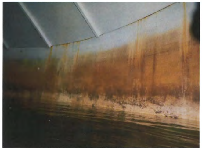
70 Top Of The Top Row Of Wall Panels At The Junction Of Where The Walls And Roof Meet Having Exposed Steel And Corrosion
