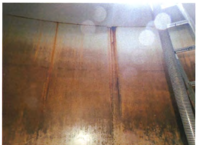
72 Top Of The Top Row Of Wall Panels At The Junction Of Where The Walls And Roof Meet Having Exposed Steel And Corrosion
